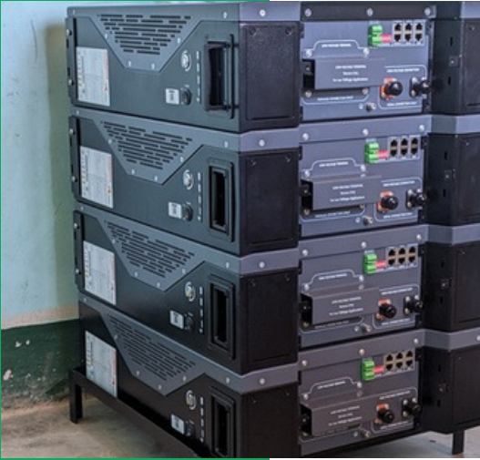
ELECTRIC BACKUP SYSTEM
