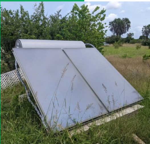
SOLAR WATER HEATING SYSTEM
